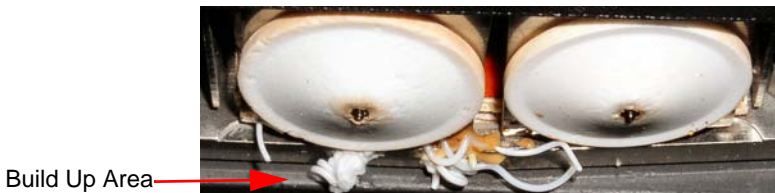
Figure 19: Material Buildup Behind Tips
